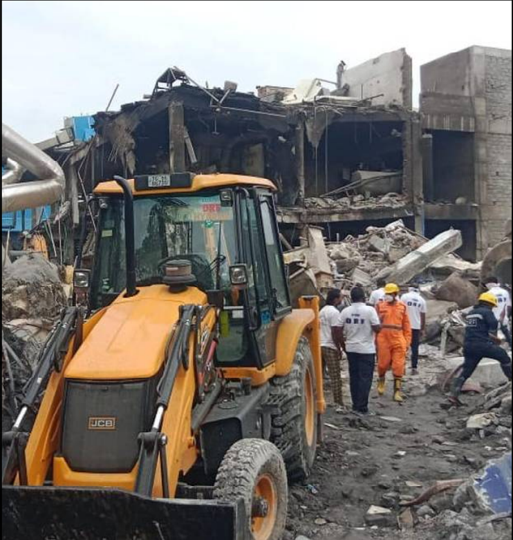
Sangareddy district, Telangana nung aliba Sigachi Industries' pharma plant nung reactor ka apokba tesem nung Fire & rescue sepaitem aliba noksa nung angur. Iba lendong ya Hombarnü atalok aser Mongolbar tashi nung iba lendong nung nisung 36 asüba jangjaogo.
